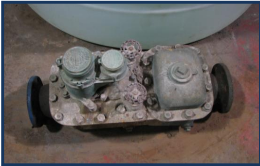
Old Meter Removed
