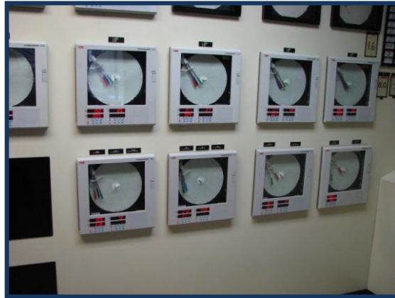
Chart Recorders in Control Room
